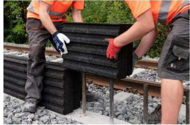
Figure 12: Example of low-height modular barriers installed in Prague.
